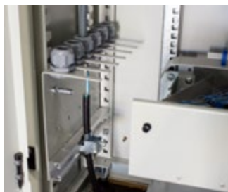
Incoming Fiber Tubes entering from the left bottom side.
