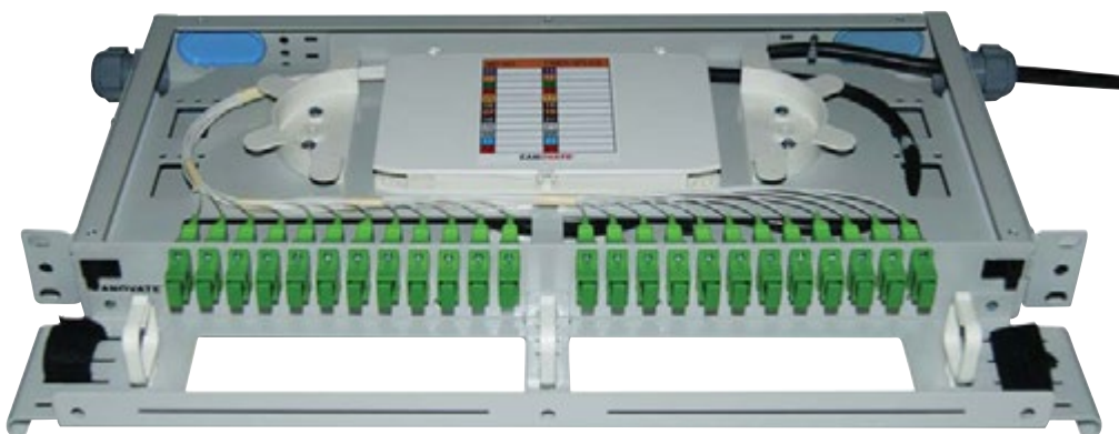
Inside view and cable management
