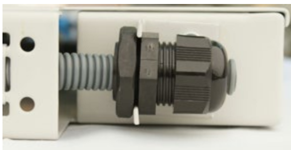
Secured cable entry
